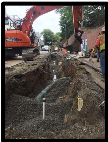
Mount Pleasant Avenue Installing 8” Water Main and 12” Drain Lateral in Front of House #40
