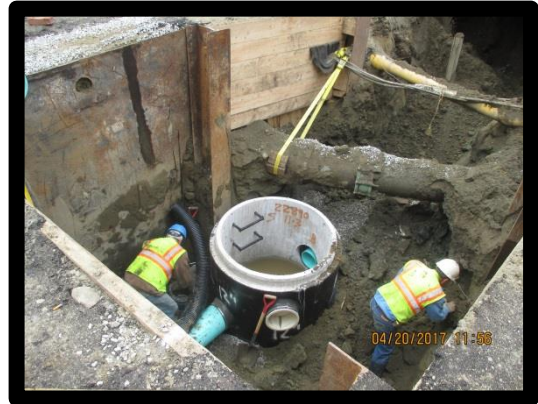
Sewer Manhole Installation at the intersection of Mount Pleasant Avenue and Forest Street
