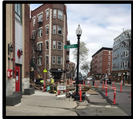
Hanover Street at Charter Street Tying-in water main in Hanover Street to Charter Street
