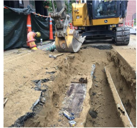
Continued Utility Conflicts Richmond Street
