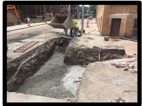
Catch Basin Lateral Installation at the Intersection of Forest Street and Vine Street
