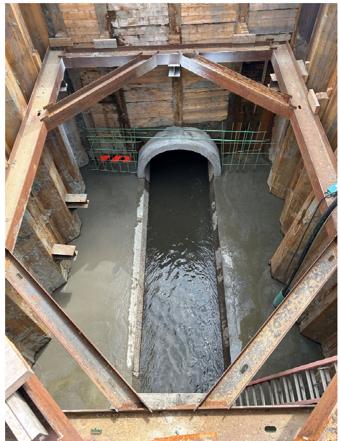
Portion of pipe was removed and working floor was poured in the jacking shaft.
