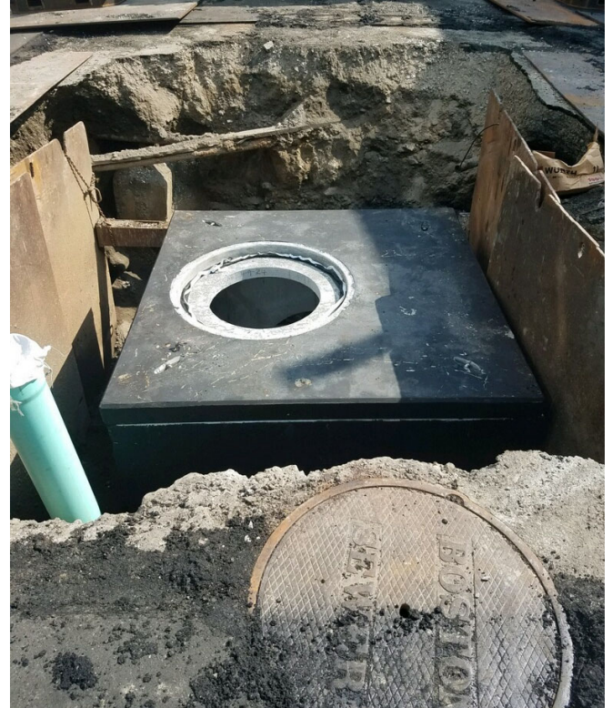
Installation of Special Manhole "B" at D Street and West Ninth Street
