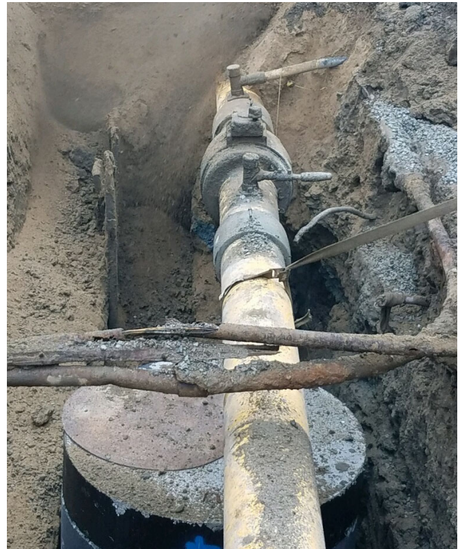
Utility congestion at a sewer manhole on D Street
