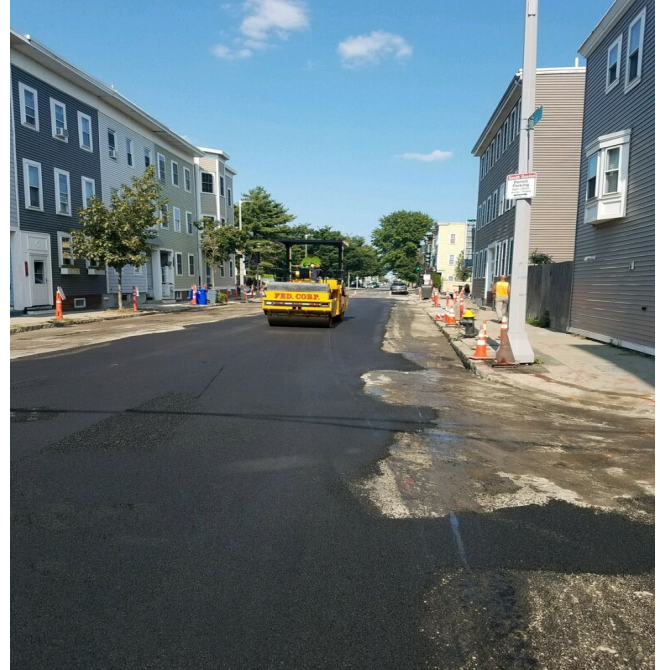
Temporary Paving Sewer and Drain Trench on D Street from Baxter Street to West Seventh Street
