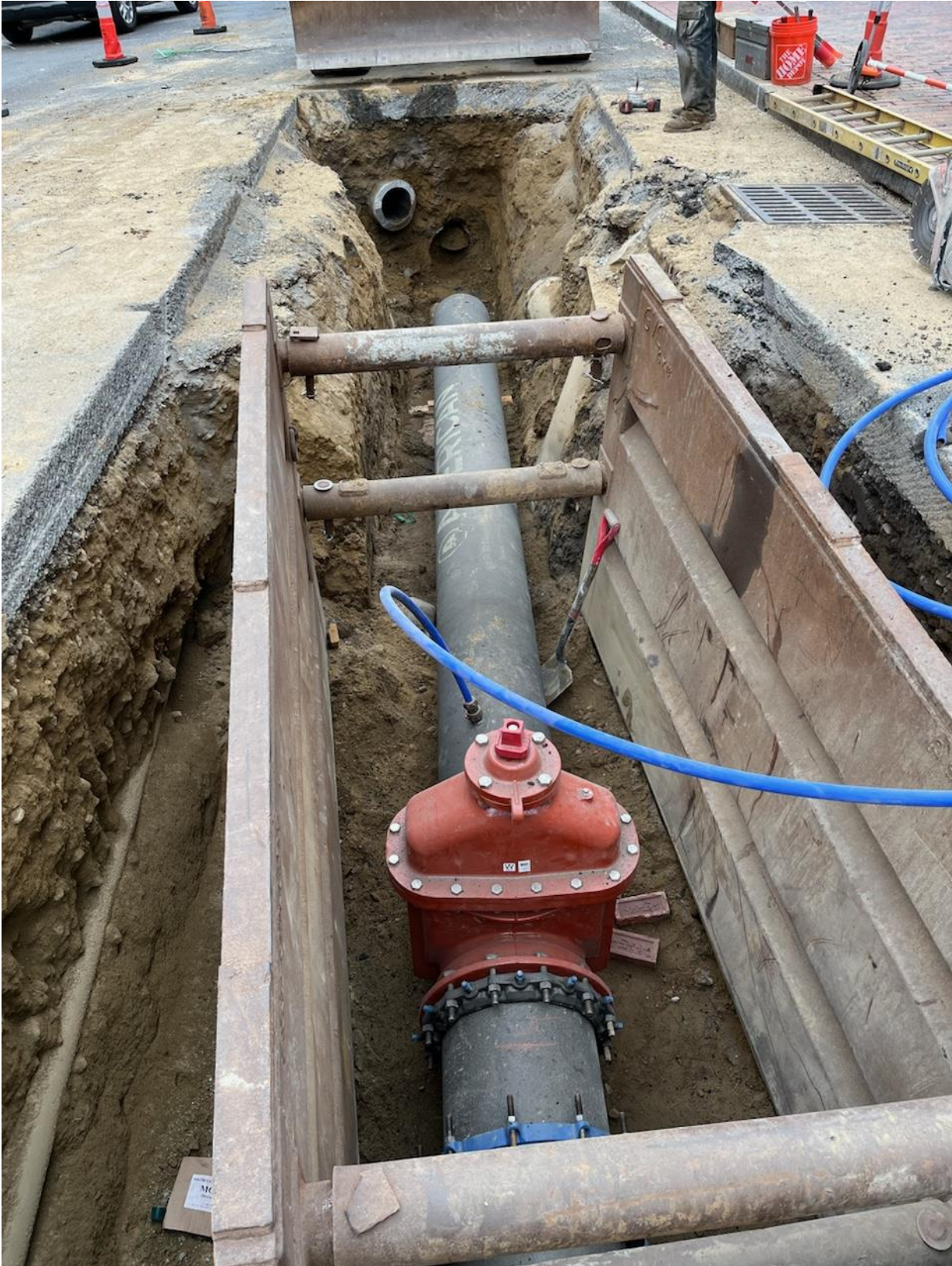
Contract 20-309-002 – Installing and preparing to disinfect newly installed water main on Park St
